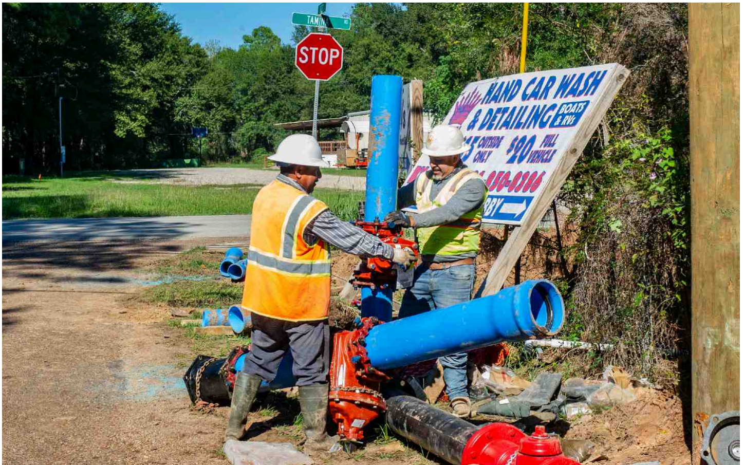
Construction personnel work with large sections of pipe for a Texas water sewer project. (Kirk Sides / Houston Chronicle via Getty Images)
